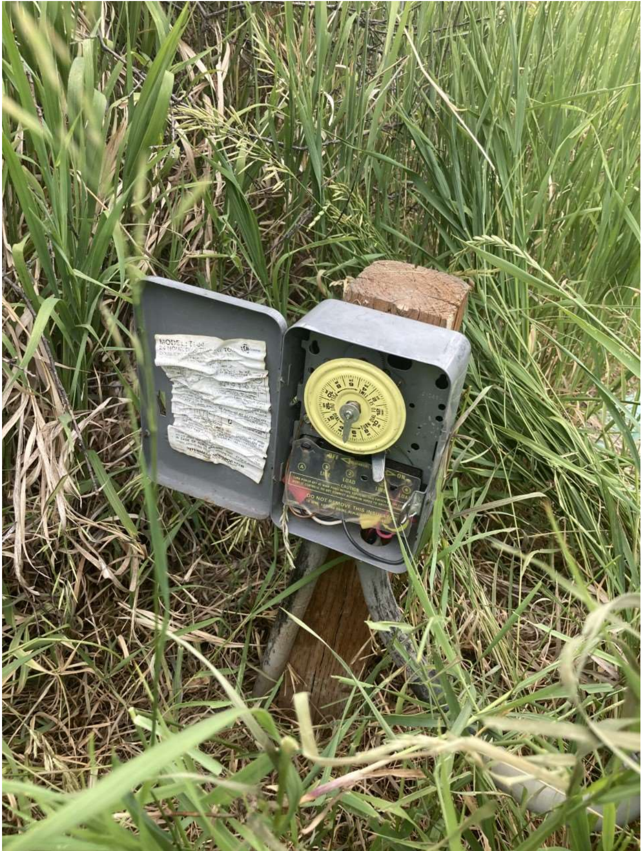
RW-2172H Breaker box 06/23/2021
